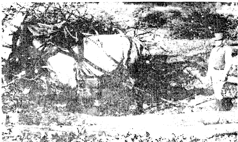
A. Ordinary reservoir clearance operations involve felling, limbing, topping, cutting, and separate piling and burning of logs and brush.
