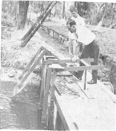
FIG. 1.—A view showing a dual tide gate installation at the end of one of the drainage ditches at the southern limit of the experimental plot. The near gate is in the "locked" position while the far gate is being held open to show the hinge action of the installation. Plot is on the left.
